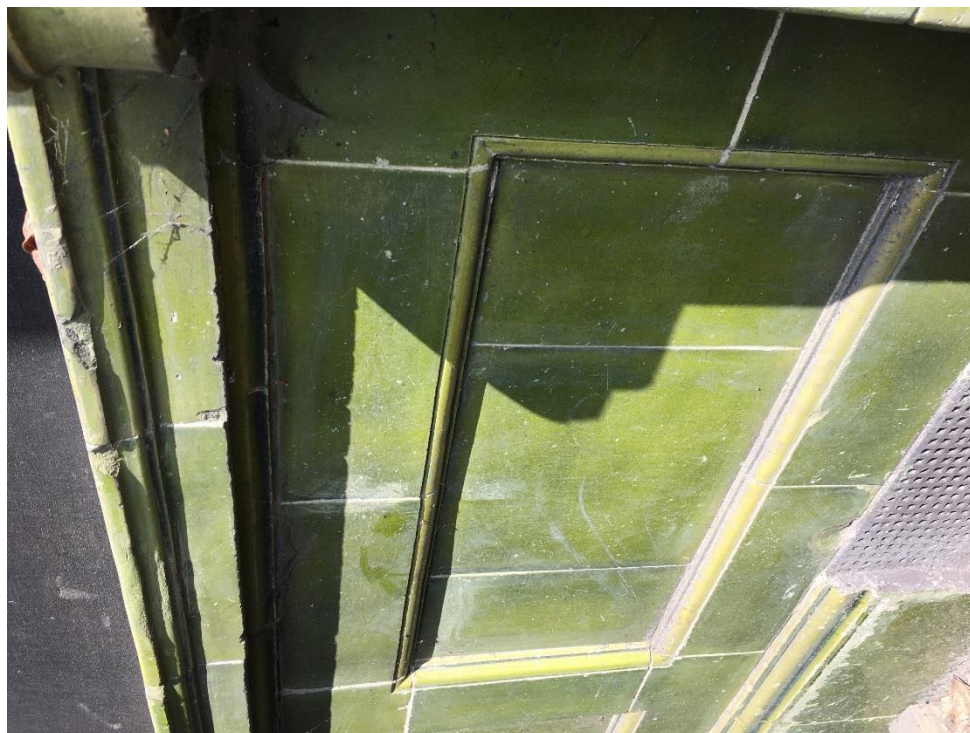
Image 10: Narrow joints between faience tiles
