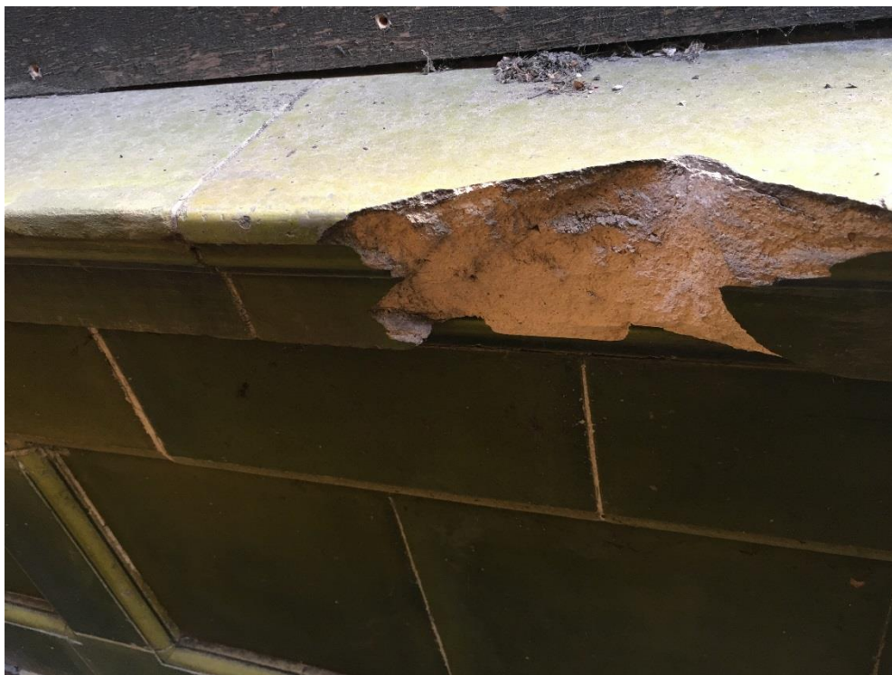
Image 11: Damaged edge showing terracotta beneath
