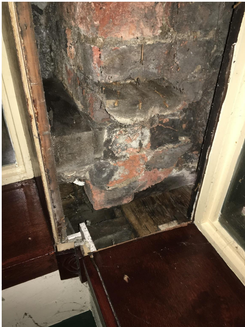
Image 5: Brickwork quality to window reveal
