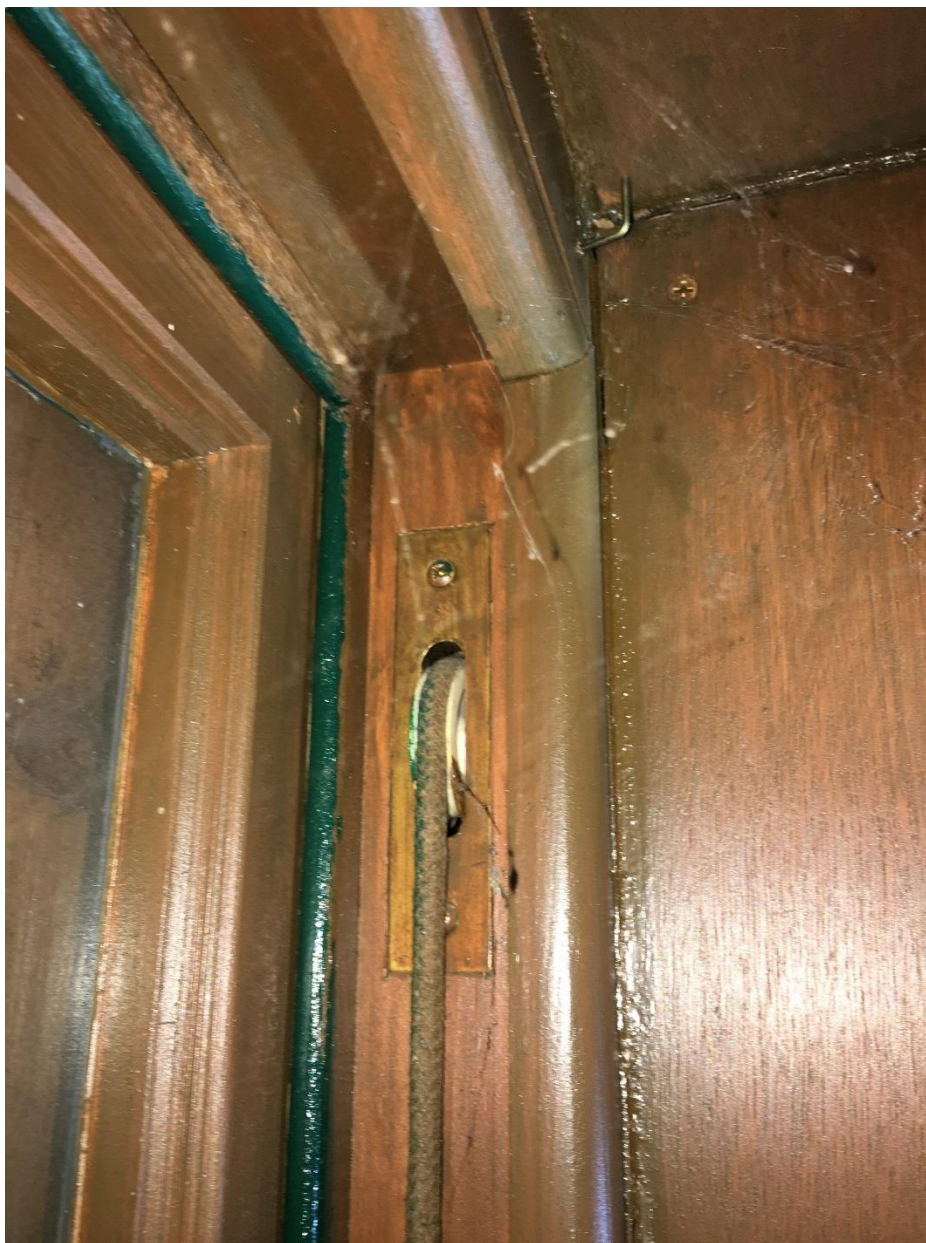
Image 3: plastic mechanism and softwood joinery to upper sash windows.
